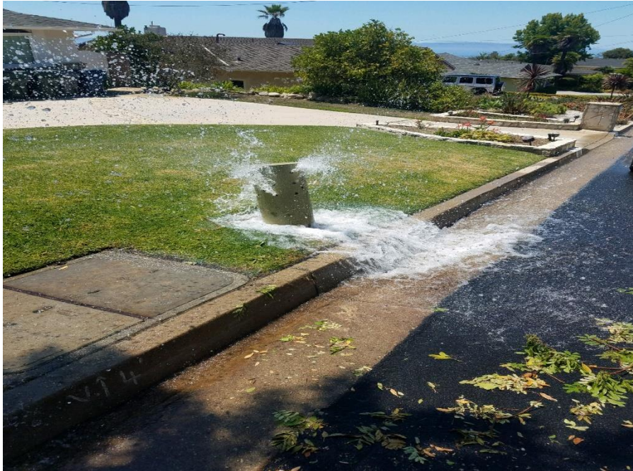
Photo of the Cal Water Leak on Corinna Drive
