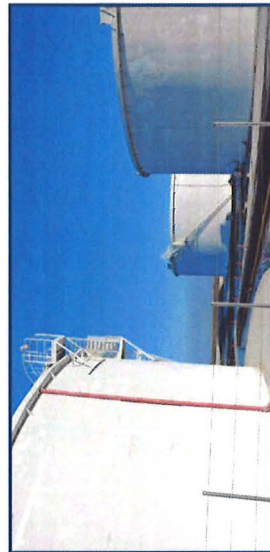
Aboveground storage tanks at the Main Terminal
